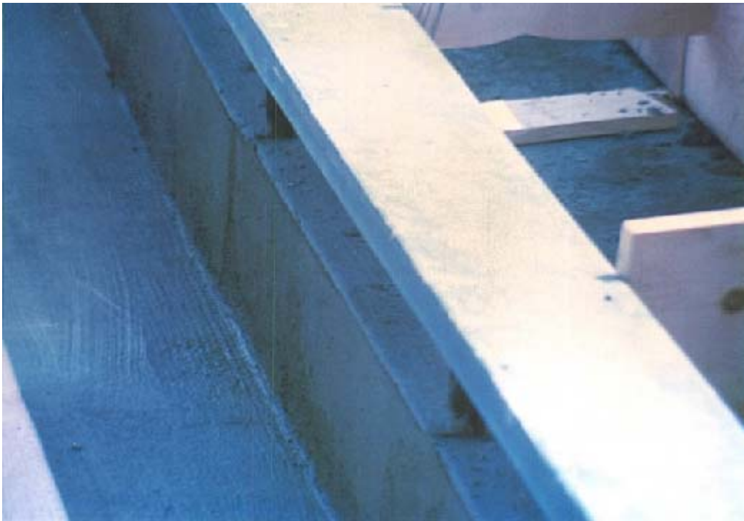
Photograph taken circa 1973 - 1974 concurrent with construction. Forming changed so that stanchions are embedded.
