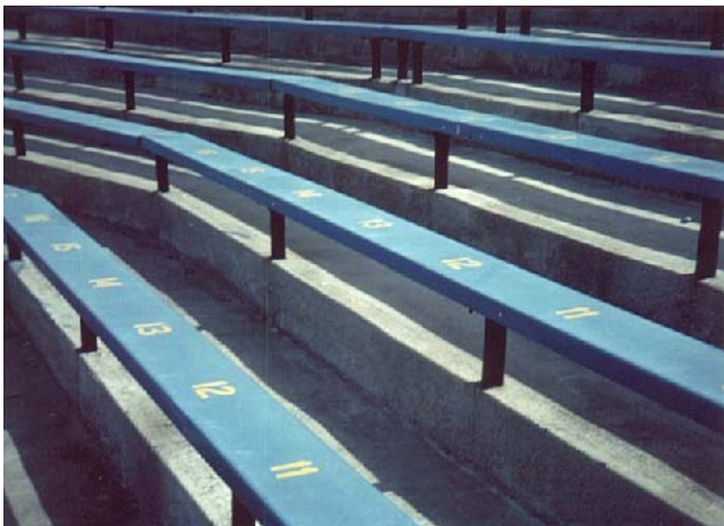
Photograph taken April 1990. Note embedded stanchions. This method was used after 1972 for the balance of the project.
