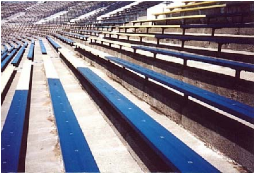
March 13, 2001 – View of east side, showing current condition of repairs done in 1970's with IPANEX Modified repair mortar.
