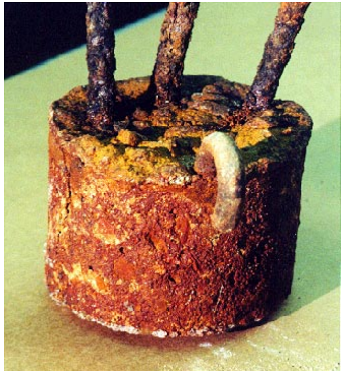
Figure 7. Photograph of IPANEX concrete after alternate exposure to 7 years 3 months in brine and 1 year 3 months in air.
